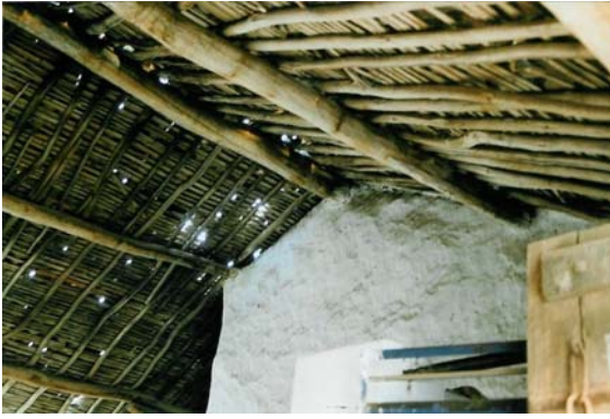
Building Construction. Fig. 14 Country tile roof from inside (photo by the author).
